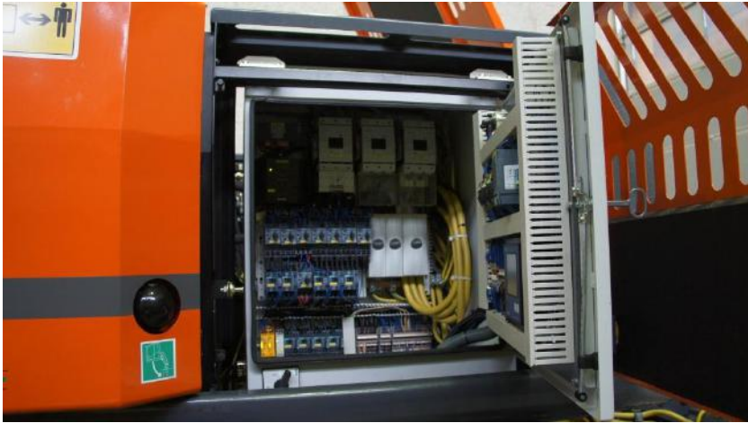
Control cabinet for E-drive
